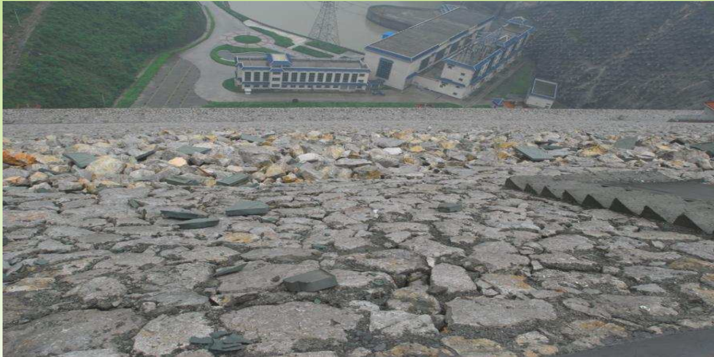
Rockfill Loosened at Upper Downstream Slope
