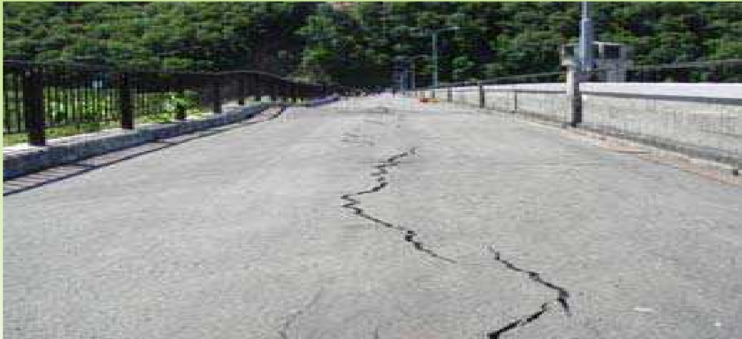
Longitudinal Crack on the Crest
