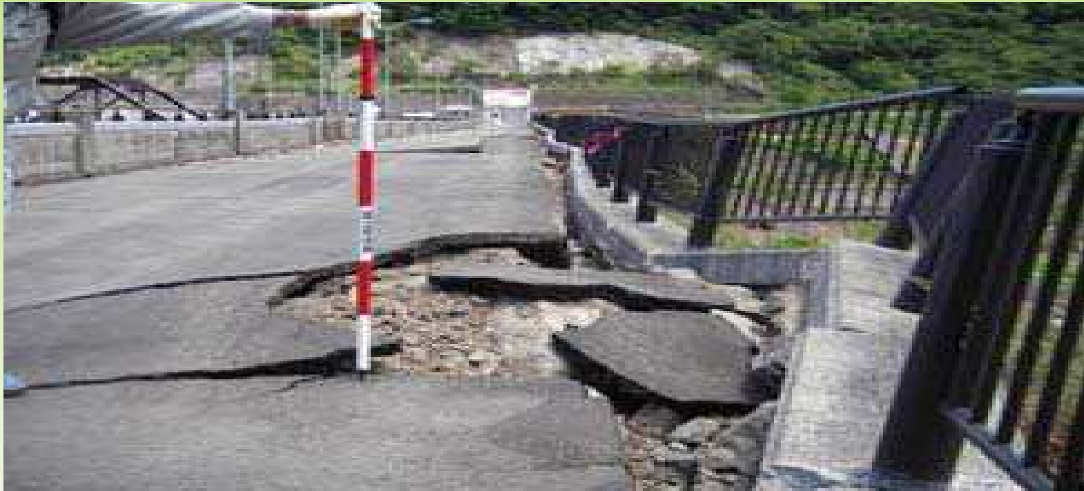
Longitudinal Crack on the Crest
