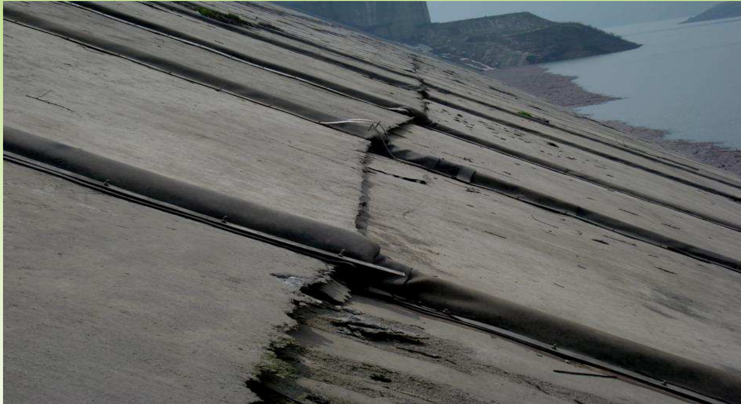
ZIPINGPU - Horizontal Joint Damaged at El.845
