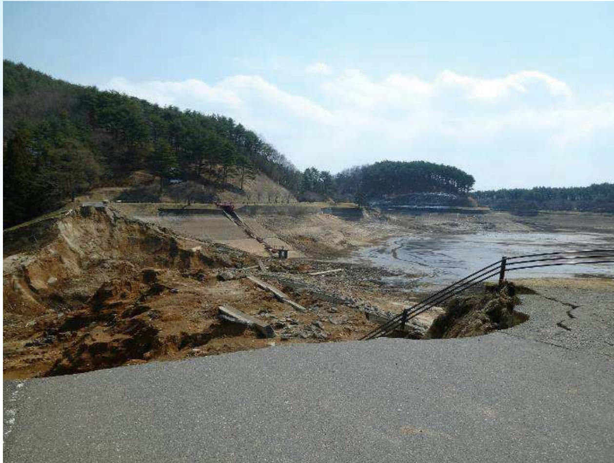
View from left abutment toward the breached portion
